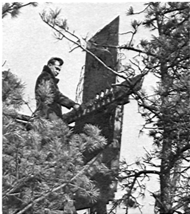
Switchboard is over 15 feet high, and concealed from the howitzer position. Simple knife switches are used for both economy and safety.
